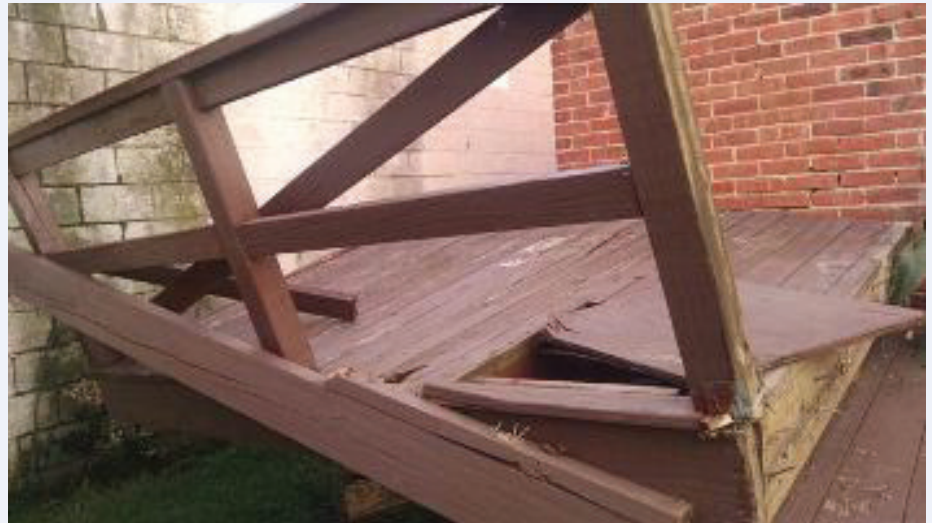
DECK COLLAPSE IN PETERSBURG
